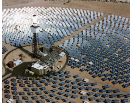
Figure 16: Example of a CSP power system (Hansen, 2016)
